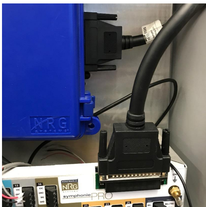
(26 Channel Wiring Panel)
