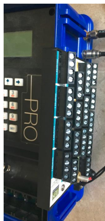
(16 Channel Wiring Panel)
