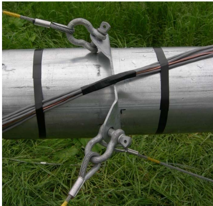
Picture 3-29: Cable protection
