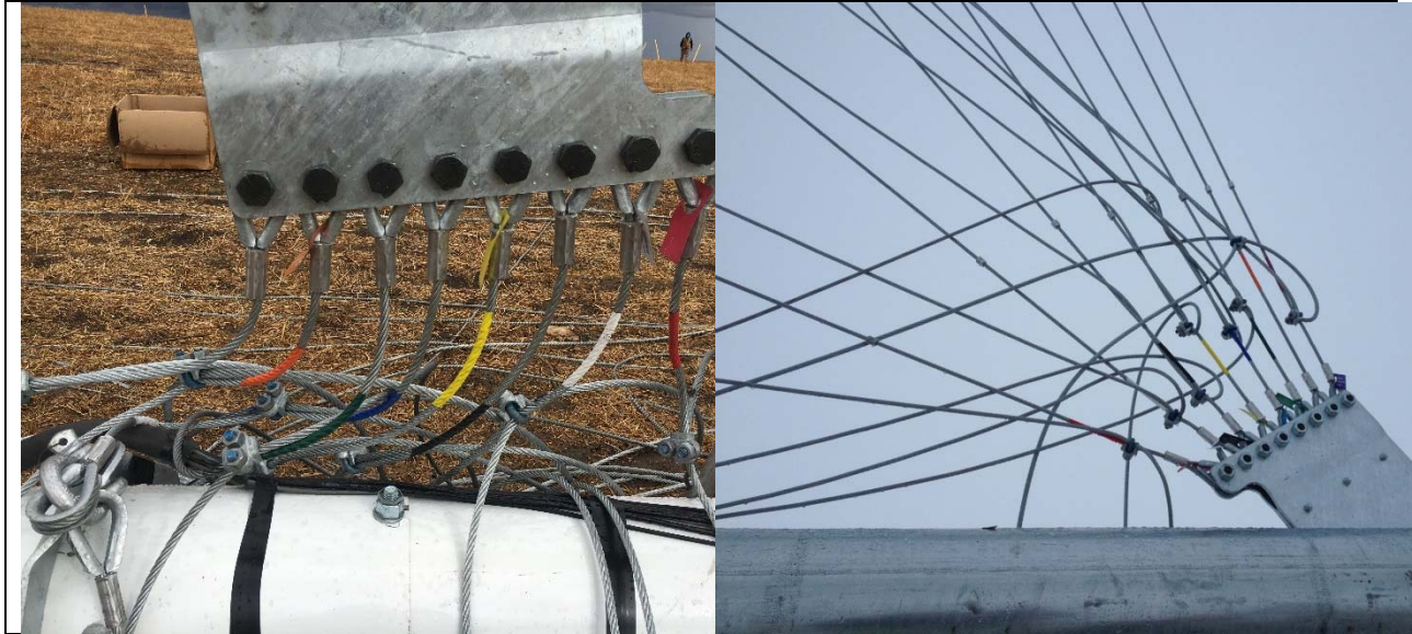
Picture 3-58: View of front guy wires attached to lifters (80 m tower) before and after tower raising
