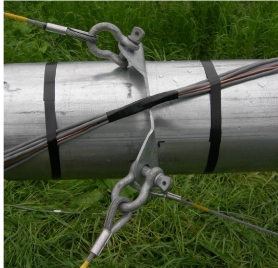
Picture 3-29: Cable protection
