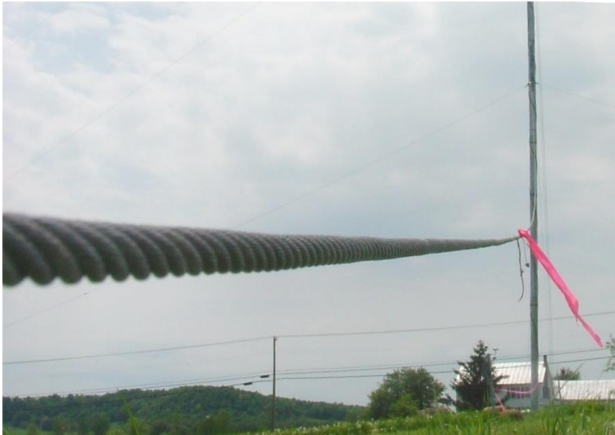
Picture 4-8: Level 1, guy sag = 2.5 tubes – TOO LOOSE!
