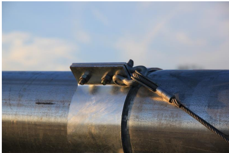
Picture 3-49: Jumper strut cable attachment
