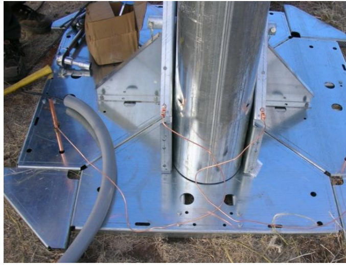
Picture 3-13: Tower Grounding
