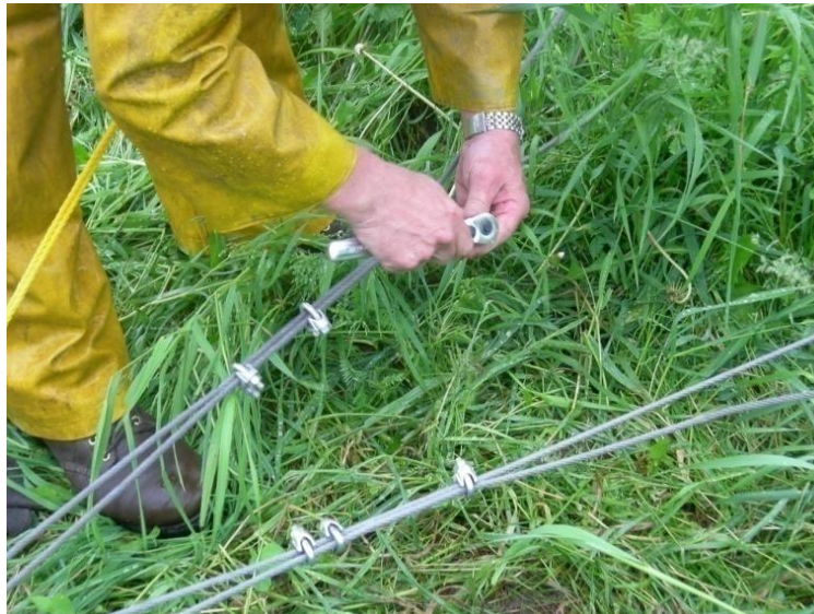
Picture 3-35: Wire rope clip guy wires together at anchor points
