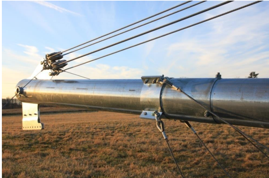
Picture 3-48: Jumper strut cable attachment
