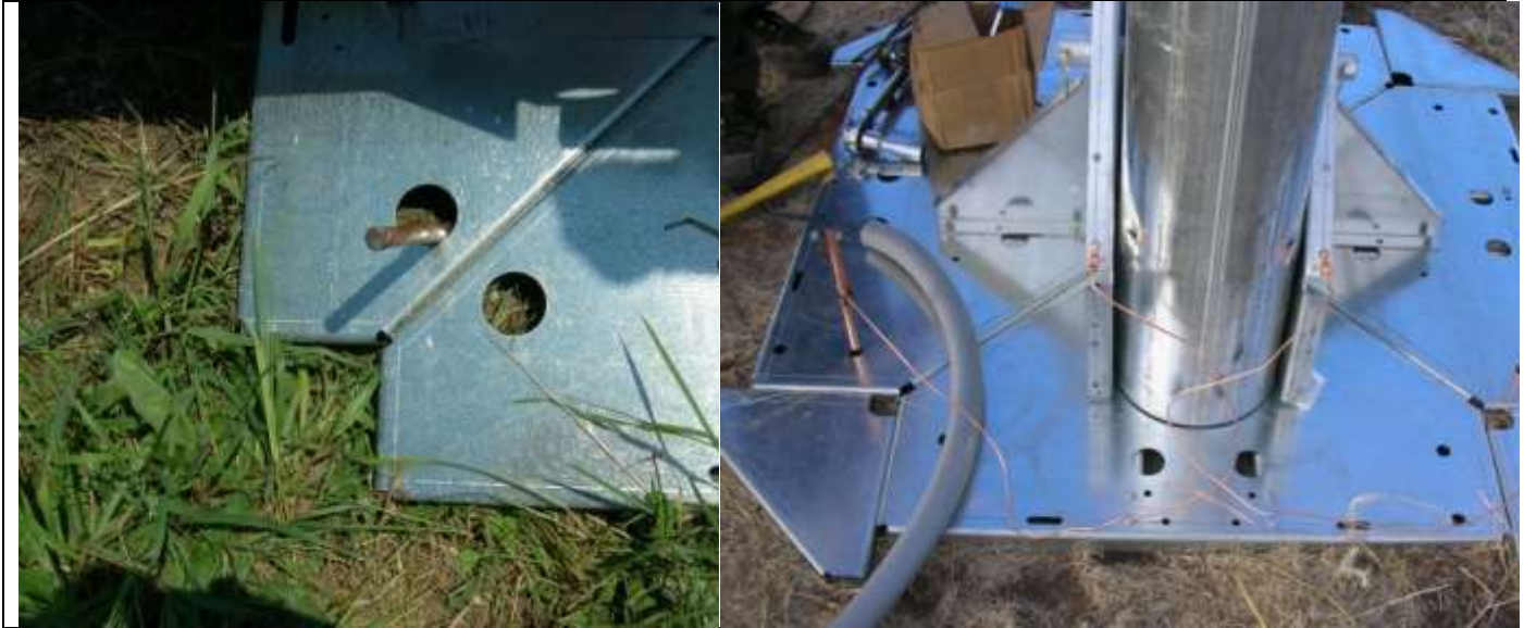
Picture 3-10 & 3-11: Grounding set-up (3-10 shows 80 meter baseplate)
