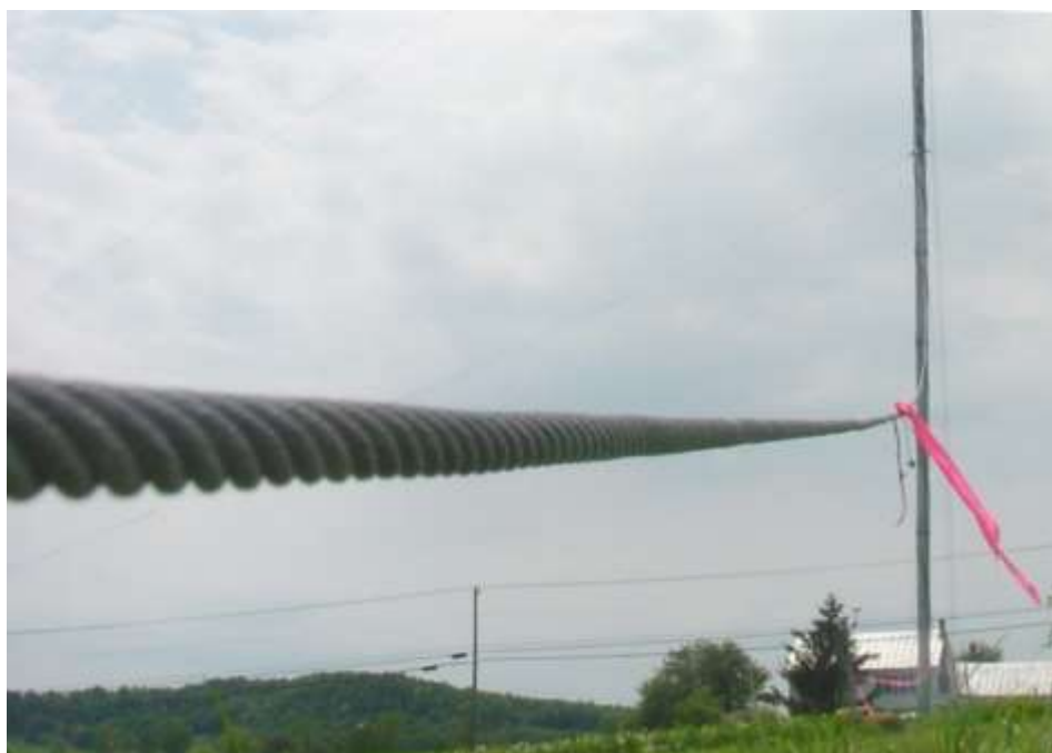
Picture 4-20: Level 1, Guy Sag = 2.6 Tubes (Too slacked)
